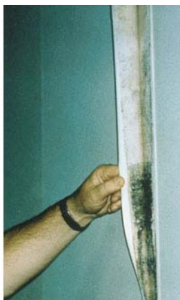
Mold growing on the back side of wallpaper.
